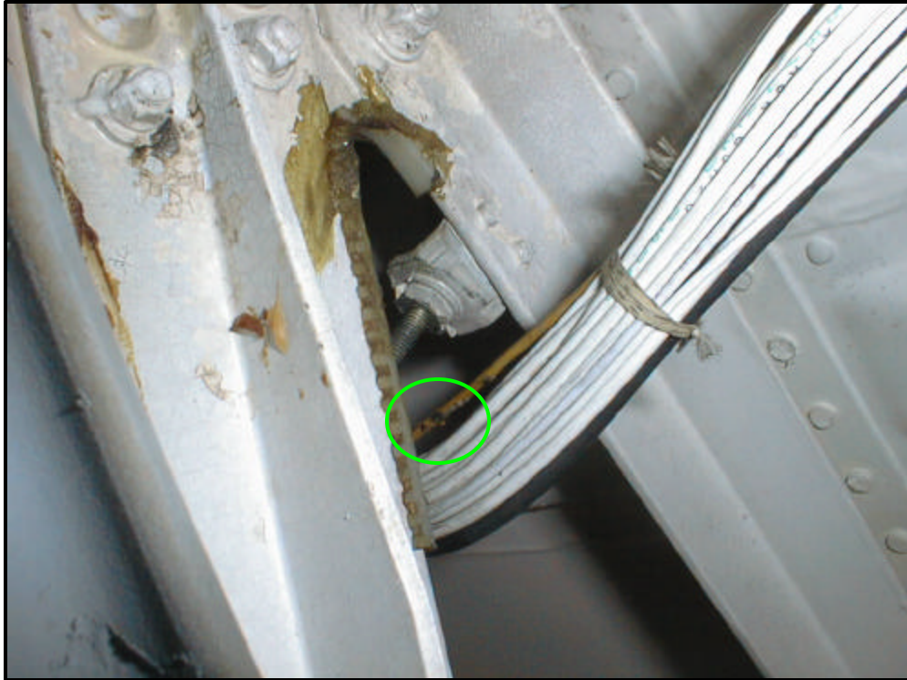
Figure 2 – Chafed insulation on Wing Tip Light Power Circuit.
